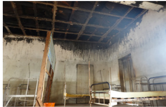
Basic infrastructure needs were identified as key to sustainable development, like the need for real classrooms (top) and repairs to health clinics (bottom).
